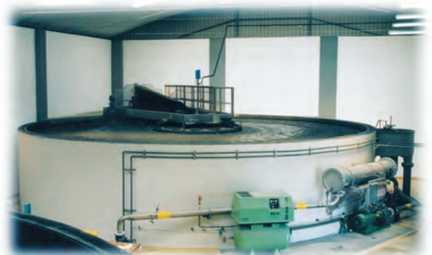
SDC 36 - Concentrating sludge from biofilter backwashing
